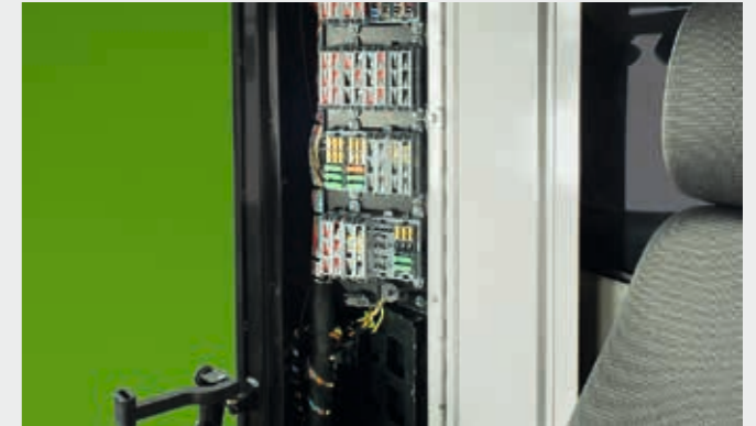
The electric fuses panel.
